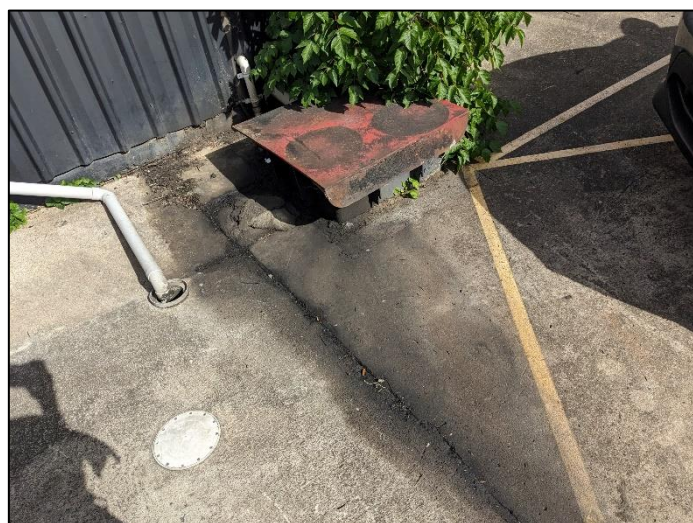
Oil-water separator presenting discolouration – AEC1
